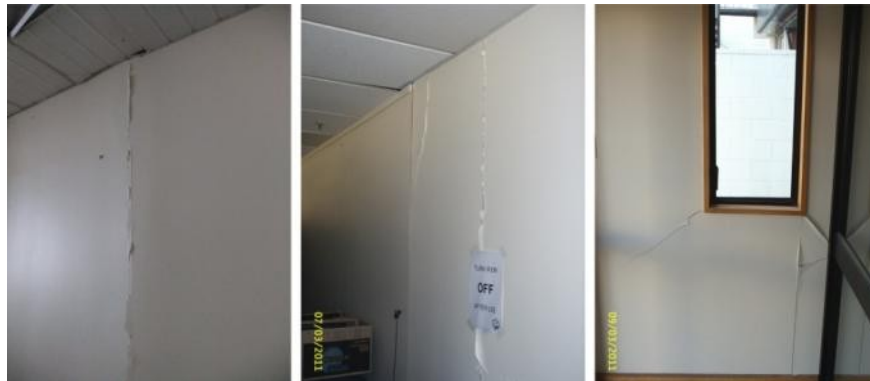
Figure 1. Typical drywall partition damage in buildings observed after 22 nd February 2011 Christchurch earthquake in New Zealand.
