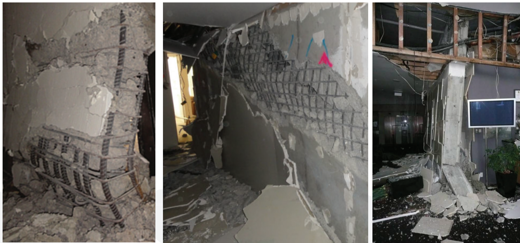
Failure modes observed in the 22 Feb 2011 Canterbury earthquake (Kam et al. 2011)
