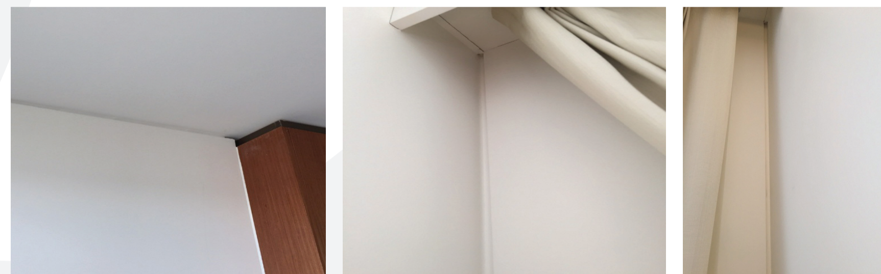
Low damage drywall application at Novotel, Christchurch (courtesy of Frank Kang, Winstone Wallboards)
