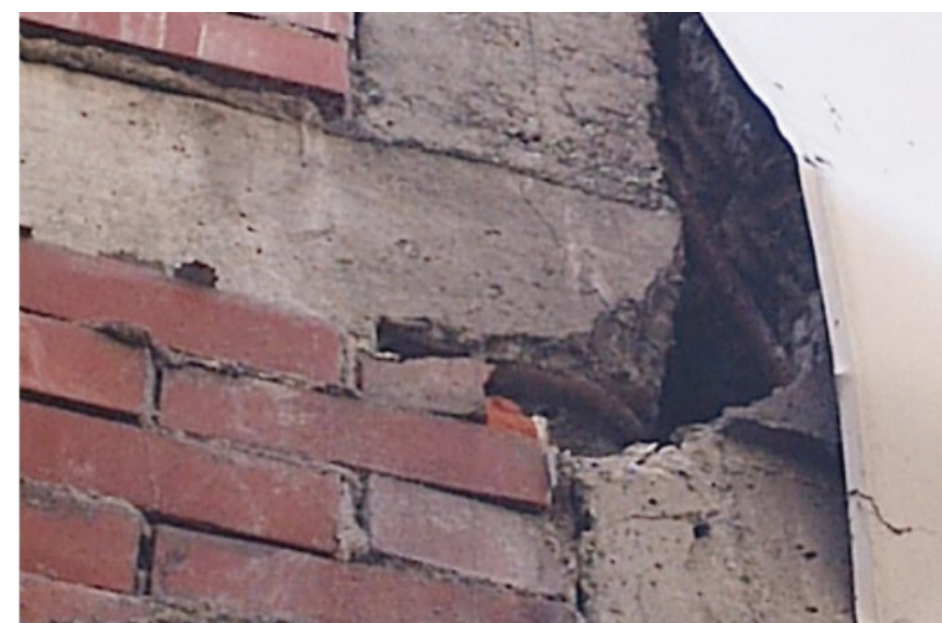
Joint shear failure (Amuri Courts, Christchurch Earthquake February 2011)
