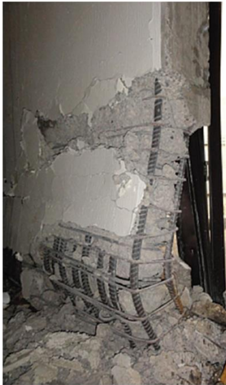
Figure 1. Out-of-plane instability of well-confined wall (2011 Christchurch earthquake) (reprinted from Kam et al. 2011, with permission from the New Zealand Society of Earthquake Engineering Inc)
