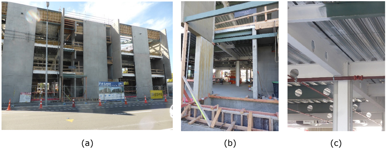
Figure 3-30: Precast concrete walls and gravity steel structure in the Forté Health building. (a) Global view, (b) Closer view of walls and gravity system, (c) Close-up of steel beams, columns, and decking
