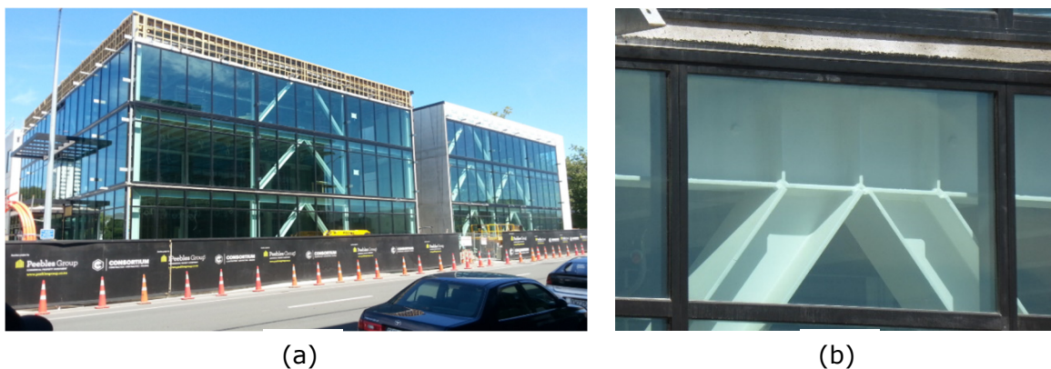
Figure 3-11: Inverted-V CBF at 124 Kilmore Street. (a) Global view, (b) Close-up of brace-to-beam connection detail
