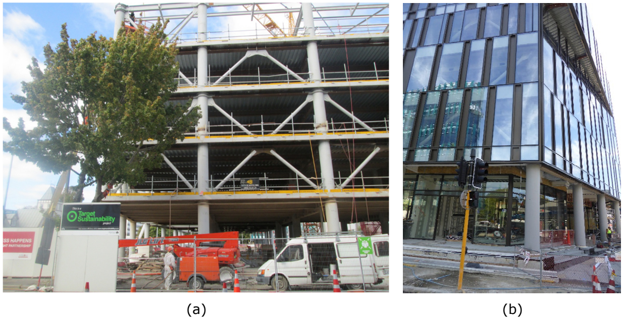
Figure 3-34: Hybrid structure example during construction, Awly Building. (a) In March 2016, (b) In March 2017
