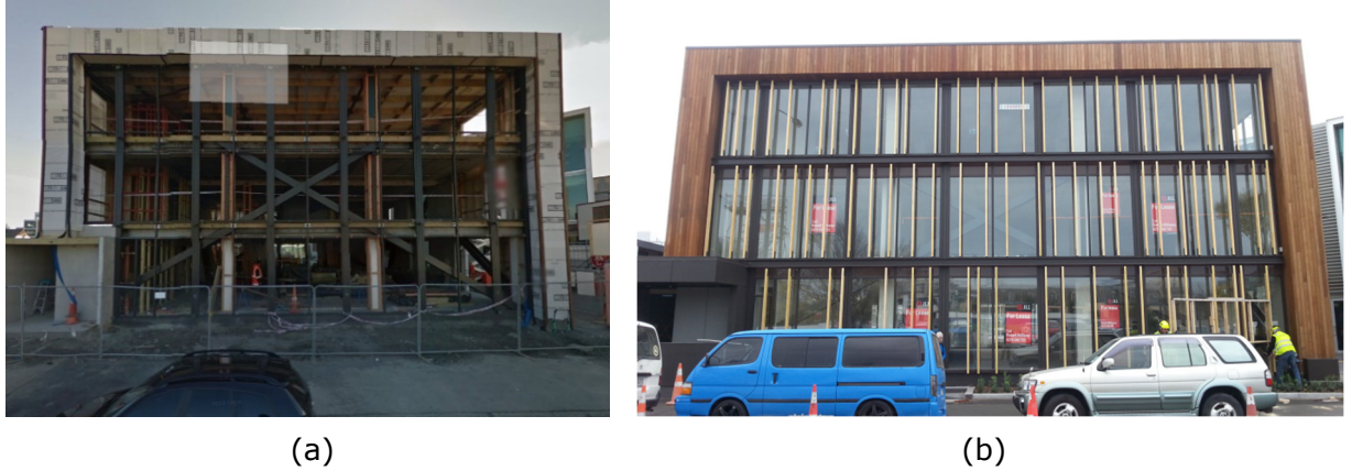
Figure 3-12: 60 Kilmore Street. (a) During construction (Google Street View, August 2015), (b) Completed, as seen May 2016
