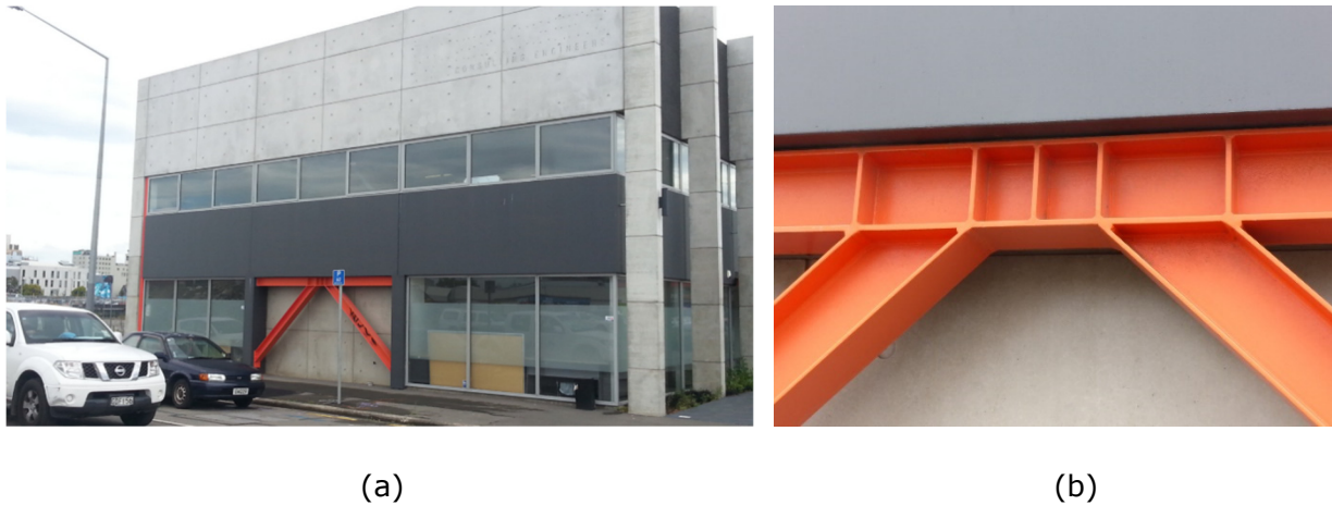
Figure 3-17: EBF, building on northwest corner of Lichfield and Barbadoes Streets. (a) Global view of inverted-V braced frame, (b) Close-up of link in inverted-V braced frame
