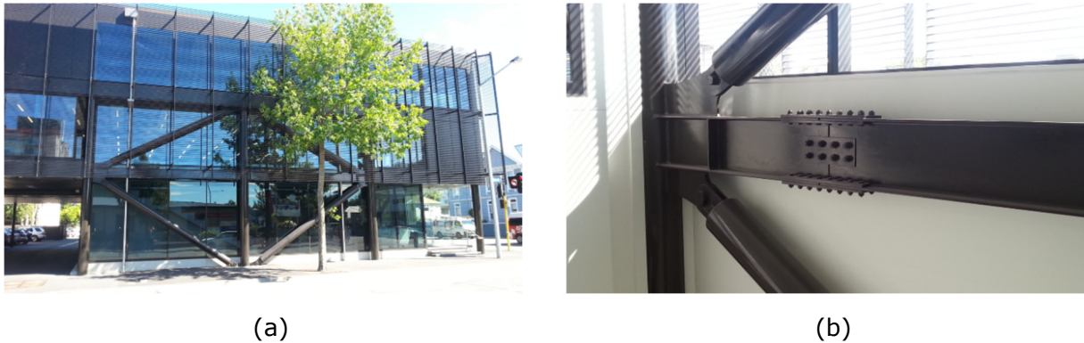
Figure 3-20: BRB frame, 254 Montreal Road. (a) Global view, (b) Close-up view of gusset connection of BRB to beams and columns
