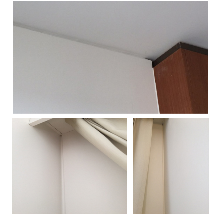
Low damage drywall application at Novotel, Christchurch (courtesy of Frank Kang, Winstone Wallboards)
