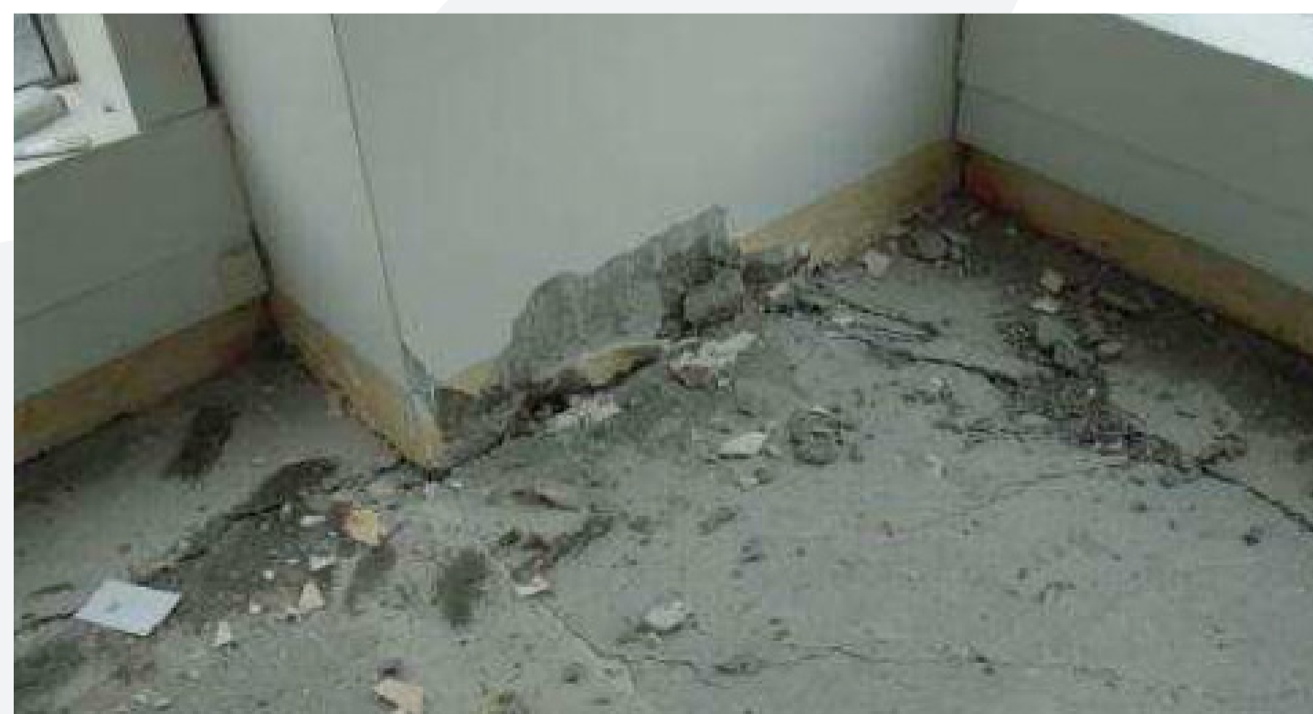
Fig 1: Damage to Precast flooring from the Christchurch earthquake. Source – Sam Corney
