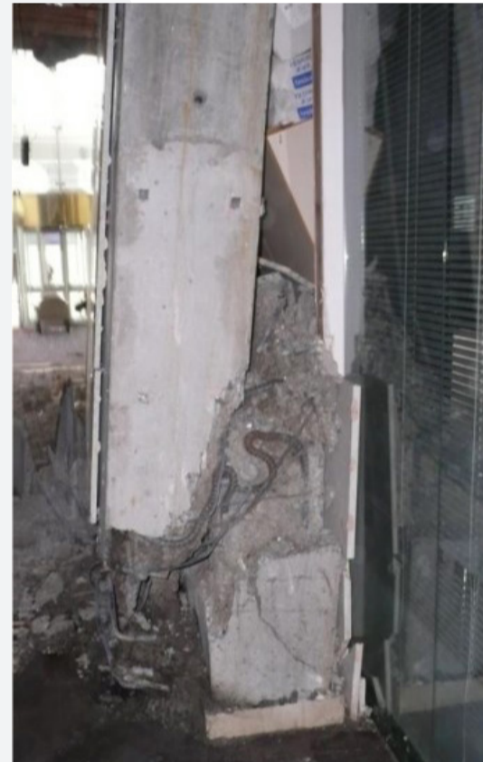
Fig 3: Axial crushing failure
