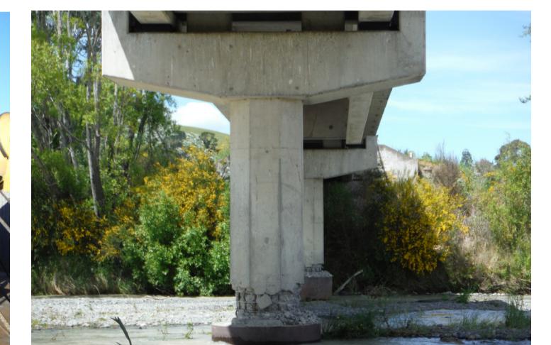
Fig 12: Damage from the 2016 Kaikoura Earthquake
