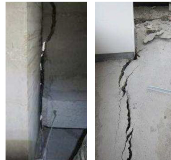
Fig 2: Damage to Precast damage. Source – Sam Corney
