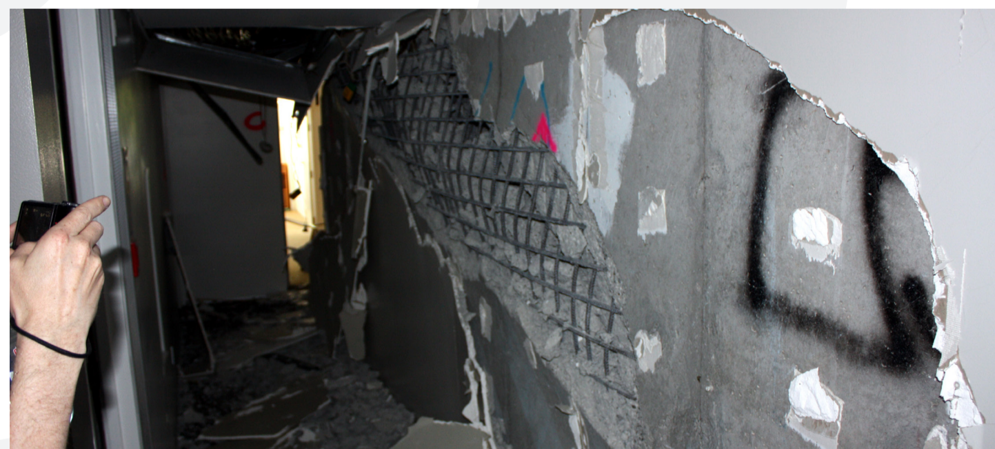
Fig 4: Web crushing failures
