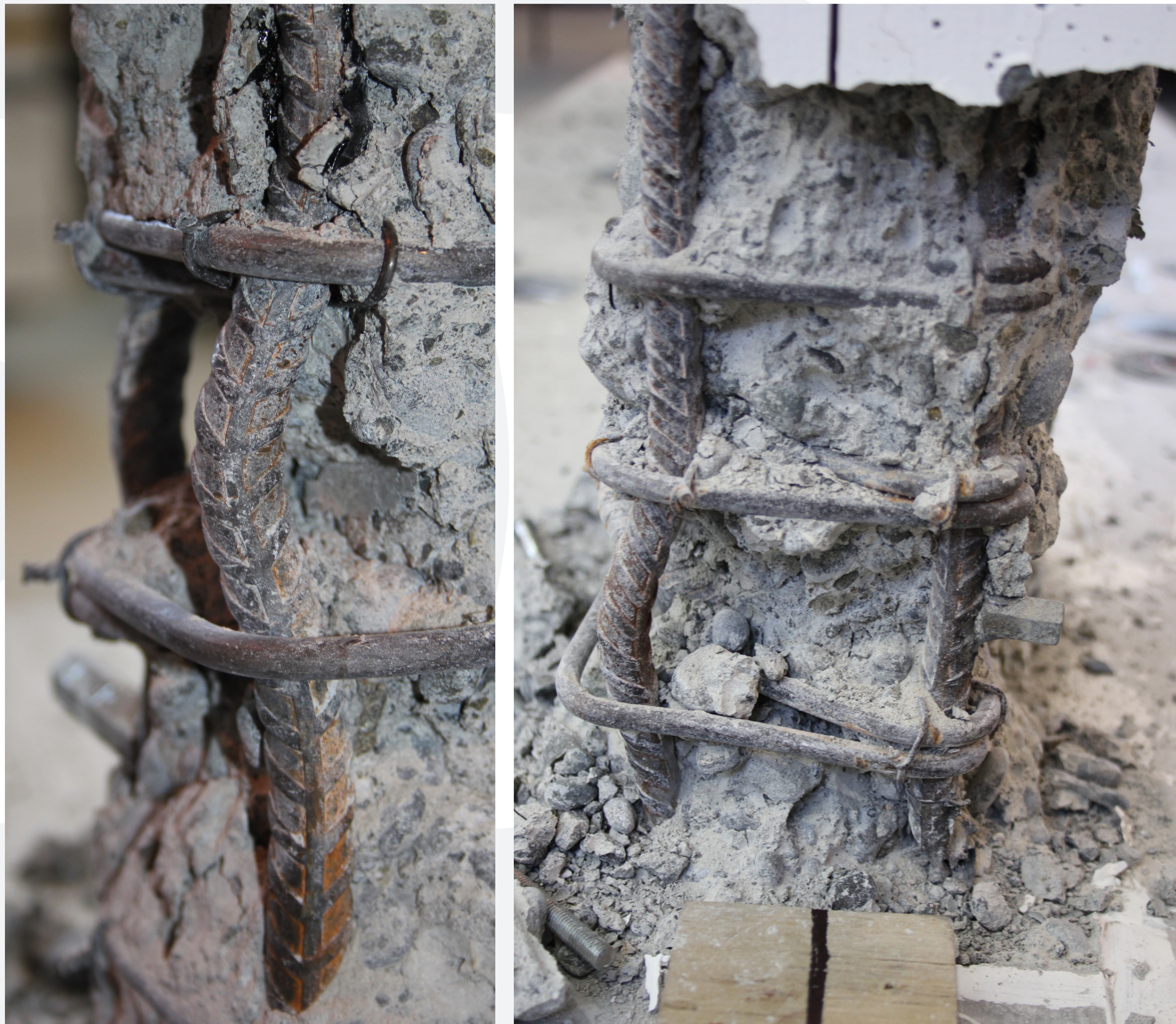
Fig 1: Bar buckling observed in the test (Dashti et al 2017)
