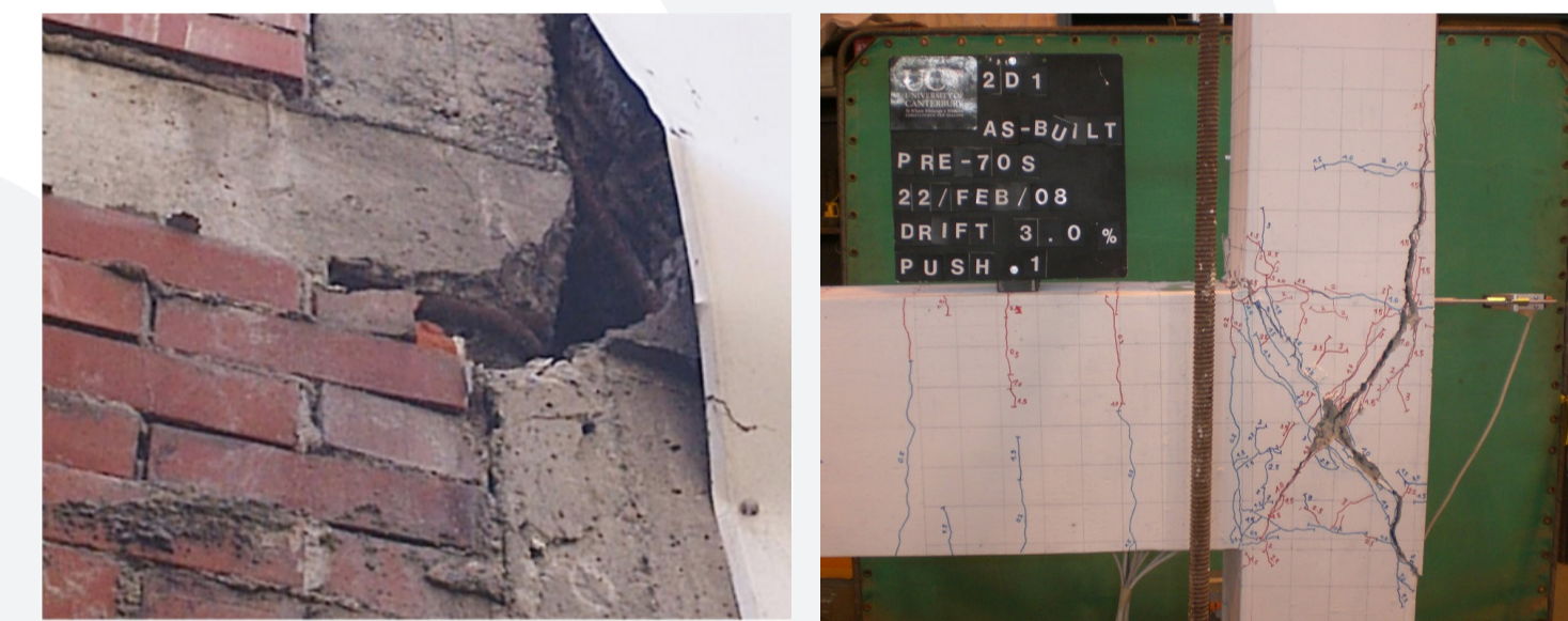
Joint shear failure (Amuri Courts, Christchurch Earthquake February 2011)
